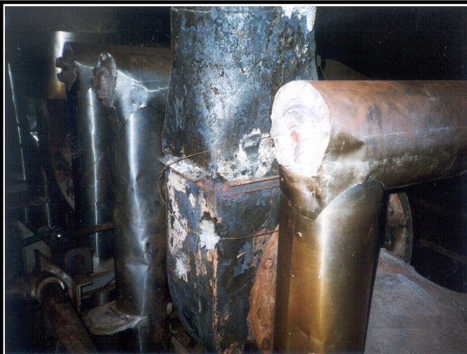
Right - An exhaust blower which has been overheated due to a radiant tube burner being out of calibration.
